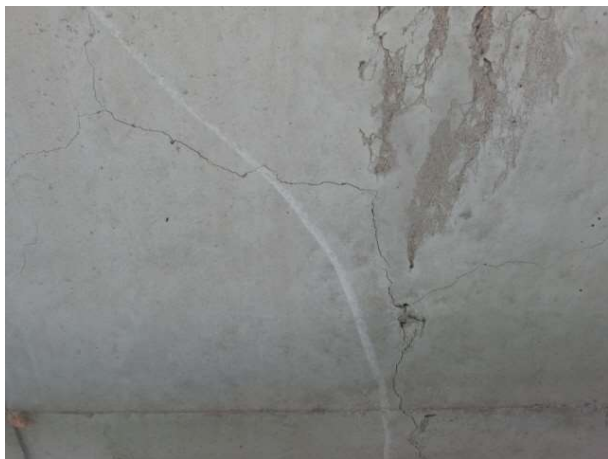
P3 코평 균열( C_w=0.2/L=1.8m )
