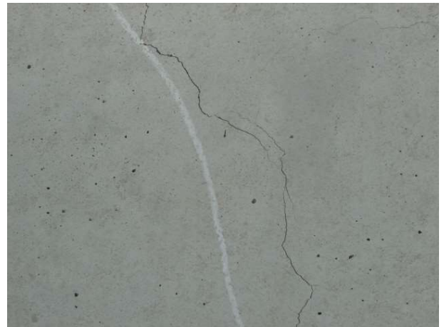
P2 코평 균열( C_w=0.3/L=2.0m )
