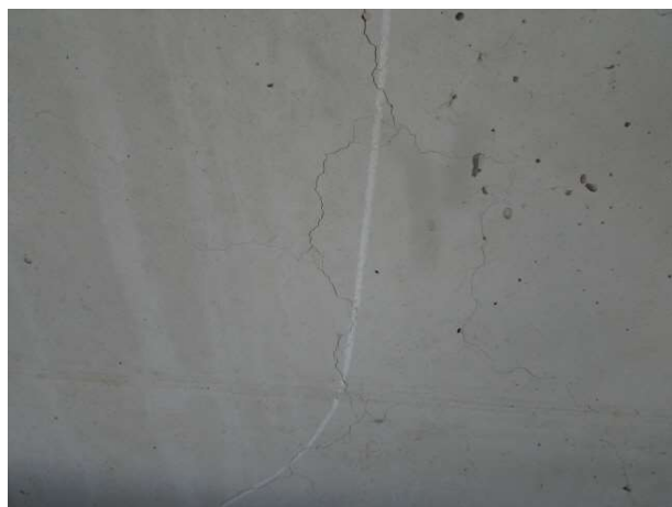
P3 코펑 균열( C_w=0.3/L=2.0m )
