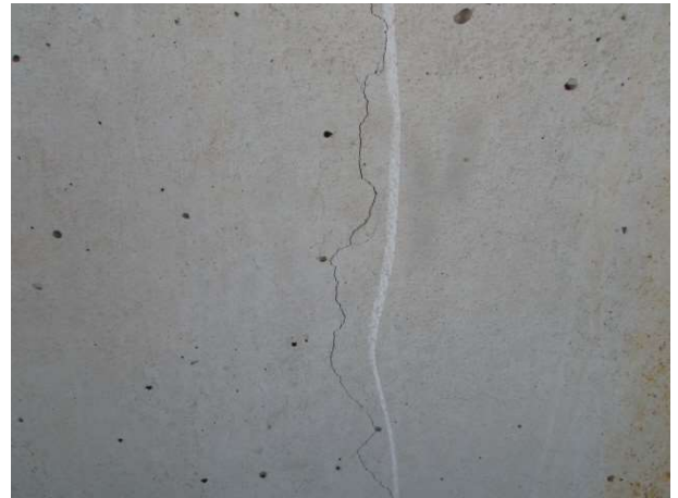
P2 코평 균열( C_w=0.3/L=1.0m )
