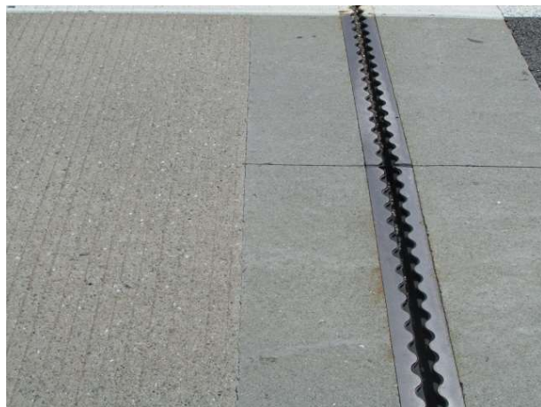
S1 후타재 균열( C_w=0.2/L=0.5m )
