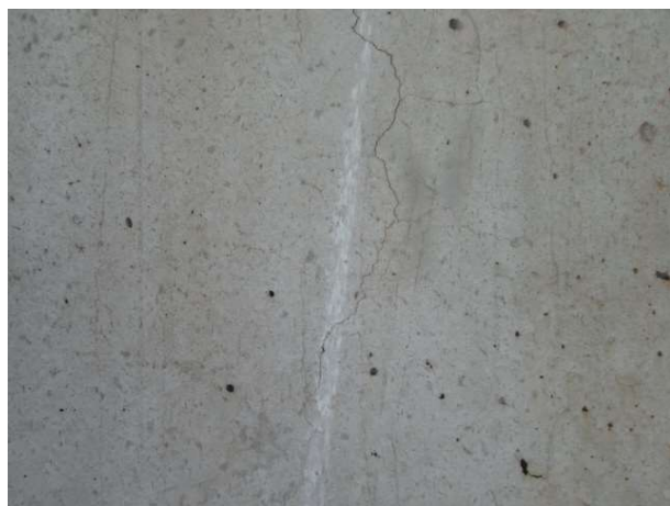
P3 코펑 균열( C_w=0.1/L=0.8m )
