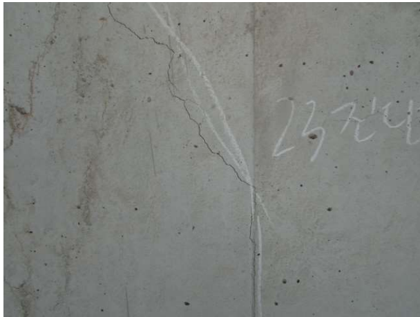
P2 코평 균열( C_w=0.3/L=1.0m )
