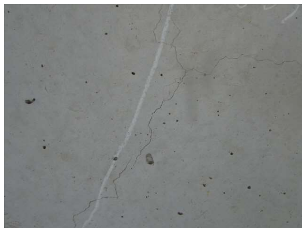
P3 코펑 균열( C_w=0.3/L=2.0m )
