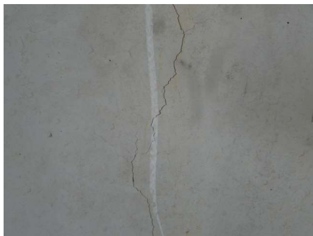
P3 코펑 균열( C_w=0.3/L=2.5m )
