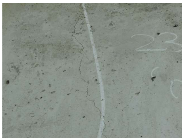
P2 코펑 균열( C_w=0.2/L=0.6m )
