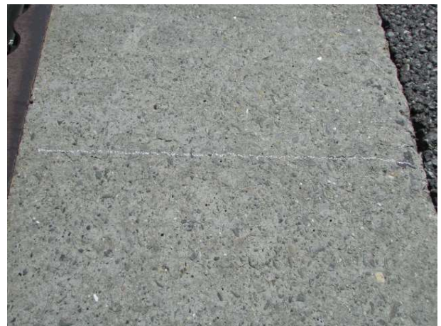
S1 후타재 균열( C_w=0.2/L=0.5m )
