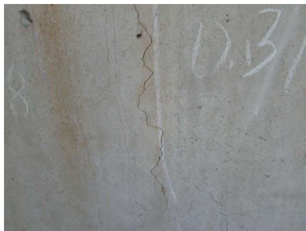
P3 코펑 균열( C_w=0.3/L=4.0m )
