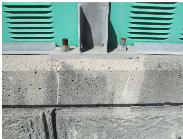
S1 방호벽 균열( C_w=0.2/L=0.2m )
