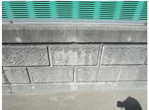
S2 방호벽 균열( C_w=0.2/L=0.6m )
