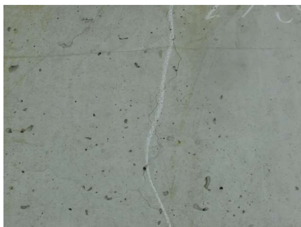
P2 코펑 균열( C_w=0.2/L=0.6m )
