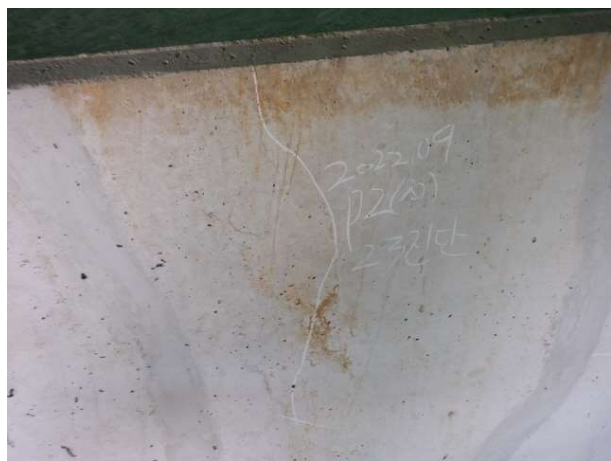
P2 코펑 균열( C_w=0.2/L=0.6m )
