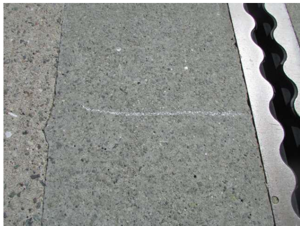
S1 후타재 균열( C_w=0.2/L=0.4m )
