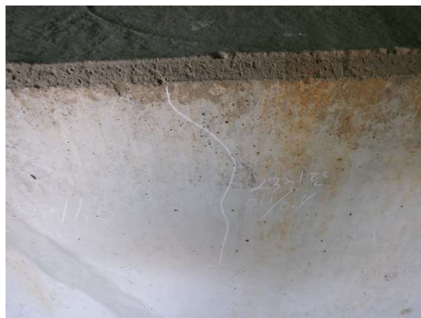
P2 코펑 균열( C_w=0.1/L=0.4m )
