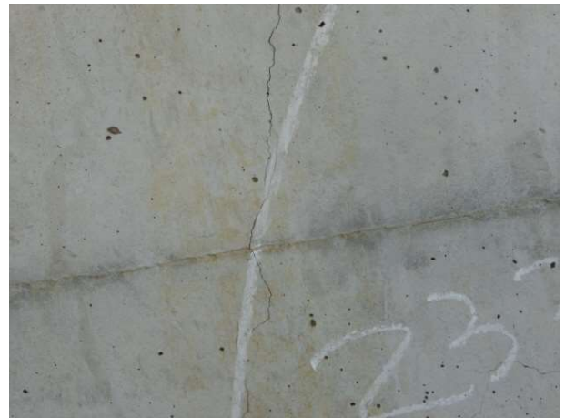
P2 코평 균열( C_w=0.2/L=2.0m )
