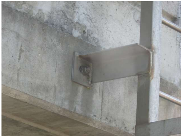
P2 코평 균열( C_w=0.2/L=1.0m )
