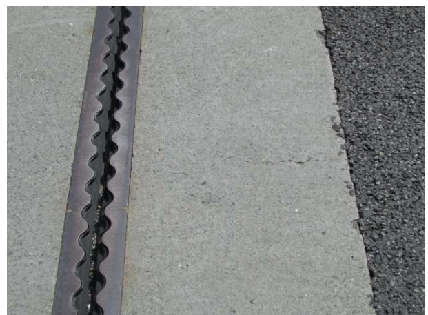
S1 후타재 균열( C_w=0.2/L=0.3m )
