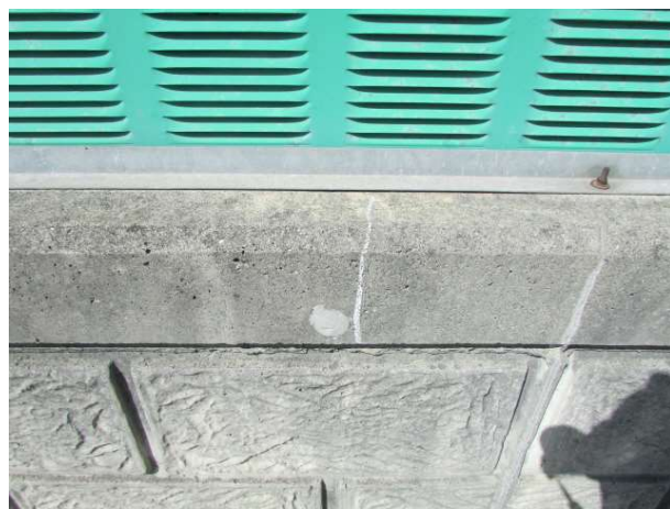
S1 방호벽 균열( C_w=0.2/L=0.3m )
