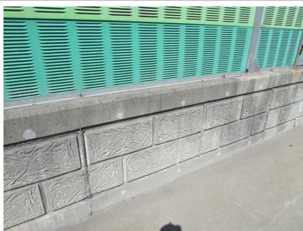
S1 방호벽 균열( C_w=0.1/L=0.6m )
