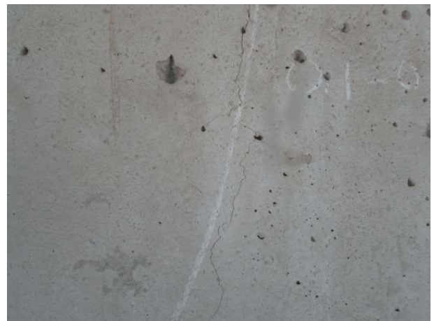
P3 코평 균열( C_w=0.2/L=4.0m )
