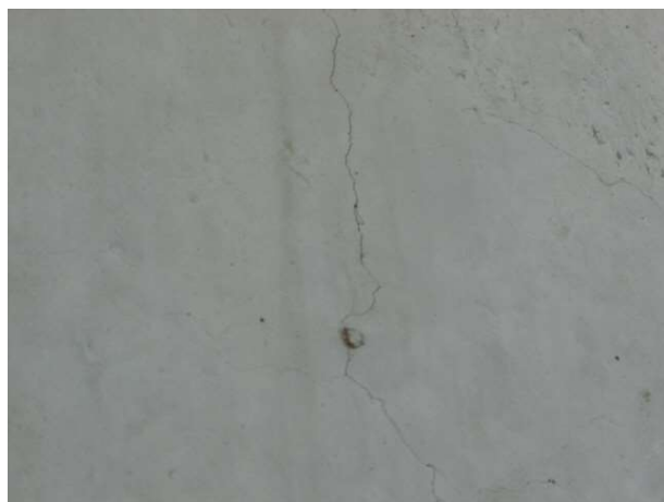
P3 코펑 균열( C_w=0.2/L=4.0m )
