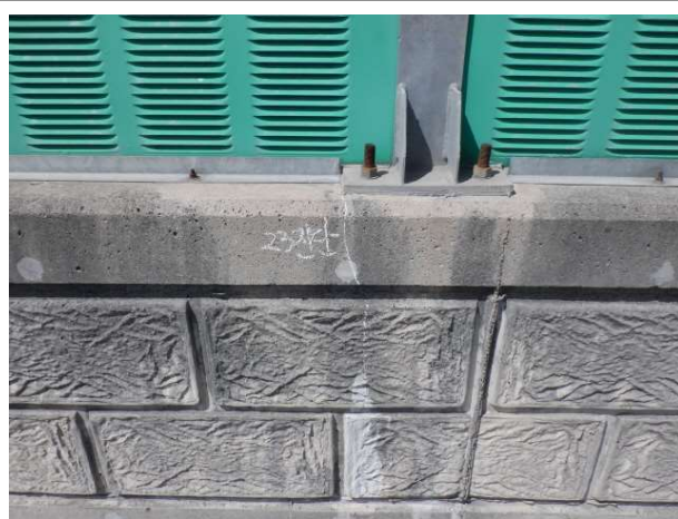
S1 방호벽 균열( C_w=0.1/L=0.5m )
