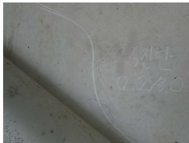
P3 코펑 균열( C_w=0.2/L=2.0m )
