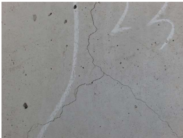
P2 코평 균열( C_w=0.3/L=1.0m )
